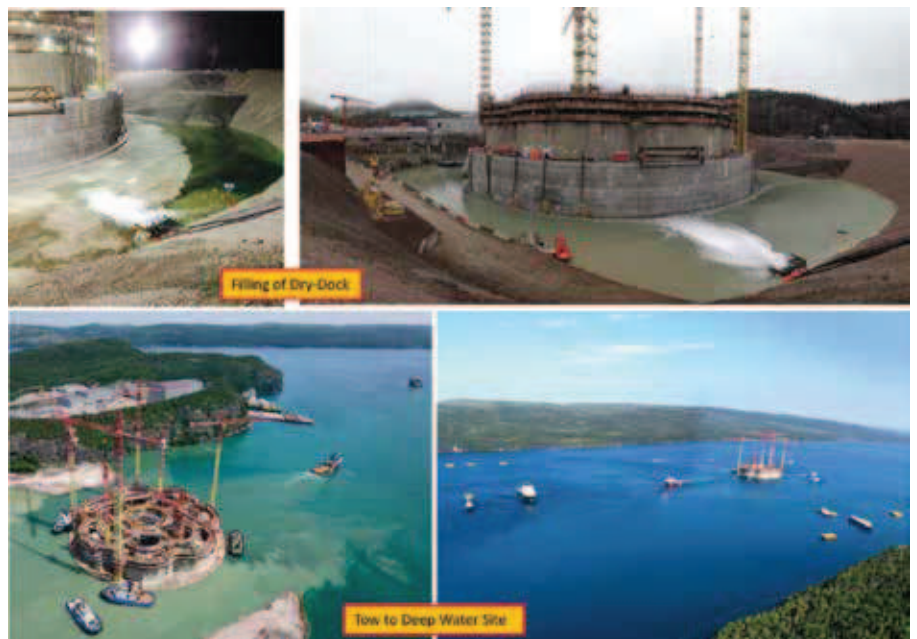
Fig. 4: After filling of the dry dock with water, the GBS was towed to the deep water site
