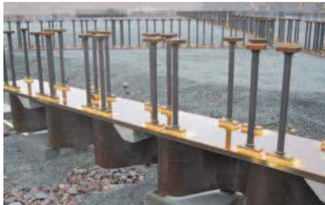
Fig. 6: Steel skirts with T-headed bars were installed below the base slab to increase sliding resistance
