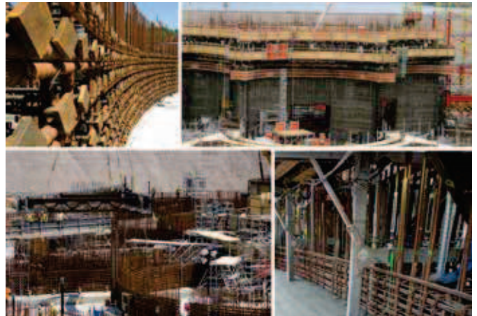
Fig. 9: Slipforming of walls with high-density reinforcement helped to minimize schedule and improve leak-tightness by eliminating most construction joints
