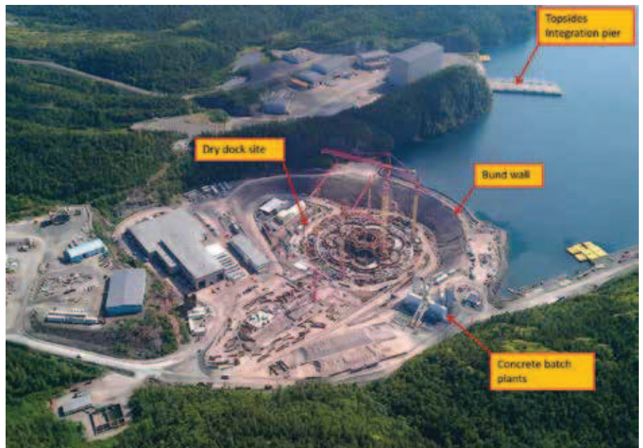
Fig. 3: The lower portion of the GBS (up to elevation of 27.5 m [90 ft]) was constructed in a dry dock created by building a bund wall and dewatering the site behind it, Bull Arm, NL, Canada
